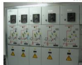
30 kV Switchgears in Subst.
