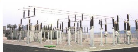
150KV Wind Farm Substation
