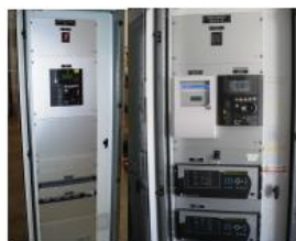
Protection Control Panel
