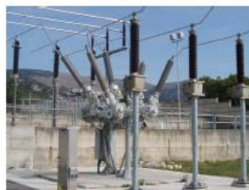
150kV GIS in Terna CP Substation
